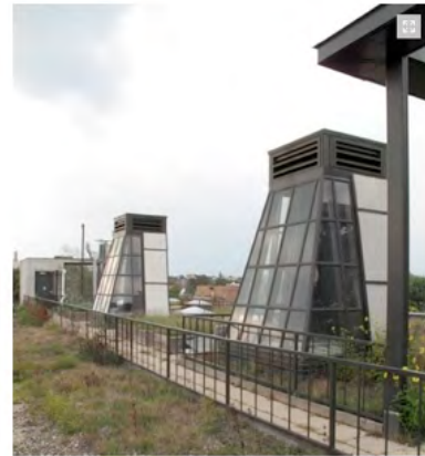
Figure 11. Solar chimneys enhance natural ventilation in the classrooms. Source: http://www.sidwell.edu/middle_school/ms-greenbuilding/index.aspx
